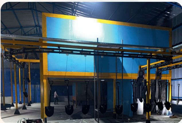
Conveyor type Powder Coating Plant
